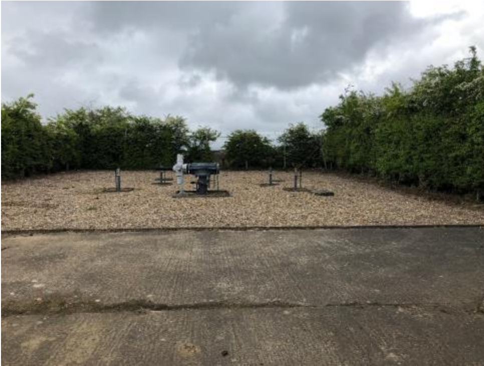
Photo 11 – National Grid Gas Valve Compound 290m west of A10 on Chequers Lane
