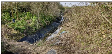
Photograph 7: Butyl-lined ditch with shallow water in some sections along the southern boundary (TN6)
