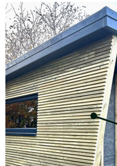
Example of horizontal pressure treated redwood (thermowood) shadow gap cladding (reference image CMR Timber Ltd)
