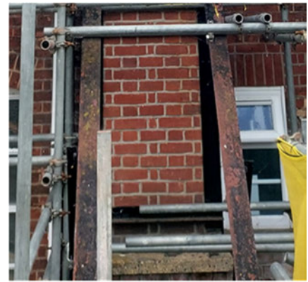
▲ Corroded steel supports
